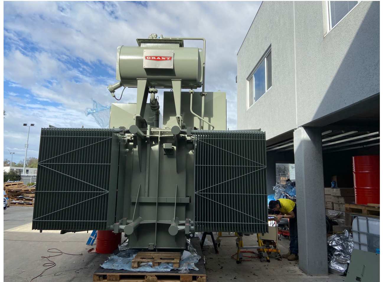
15MVA 33000//11000 Oil Cooled Power Transformer
