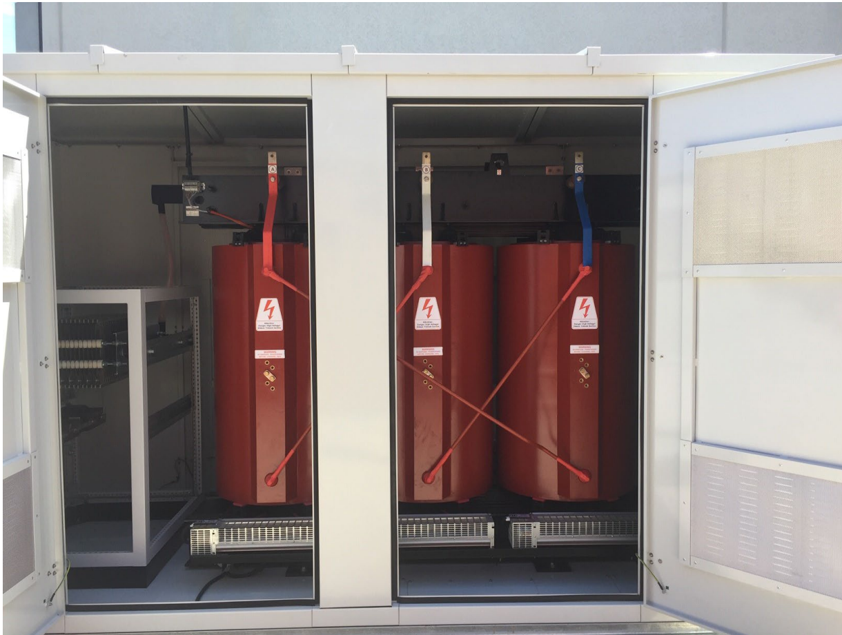
Outdoor Dry Type Cast Resin 2.6MVA 11000/3300V Dyn11 AN/AF IP44+Neutral Earthing Resistor (NER)
